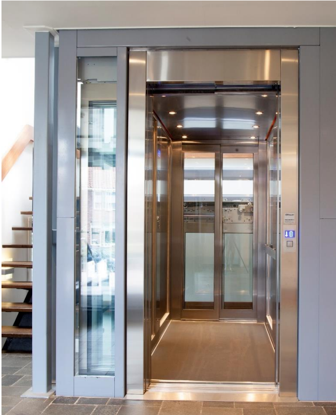
Hospital medical center Baarn, Netherlands
